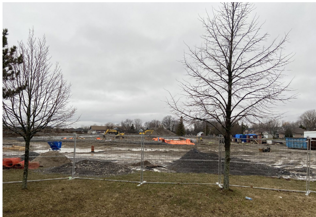
With the spring thaw underway, activity will begin at the Centre for Life construction site
